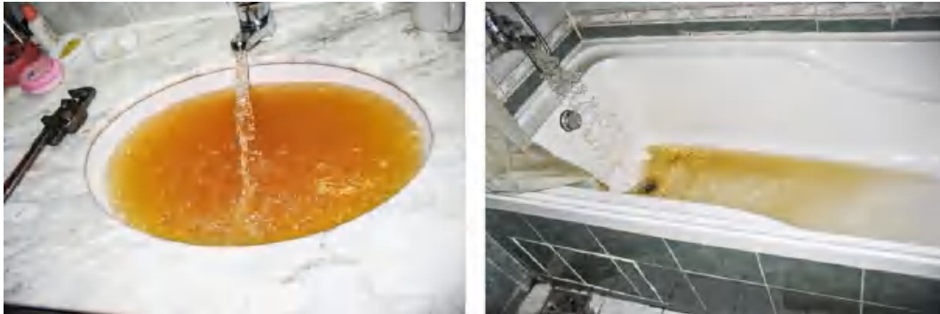
Rust condition of the guest room bathroom on the day of installation
